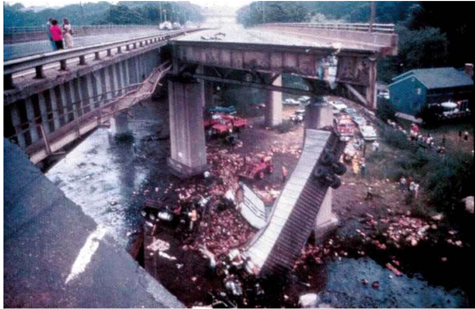
Figure 1.2.1 Mianus Bridge Failure
